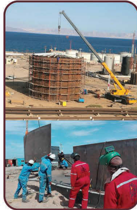
Construction of Crude Oil Tank & Water Tank (2000 m3/ Tank) Ras Ghareb - Red Sea - GPC
