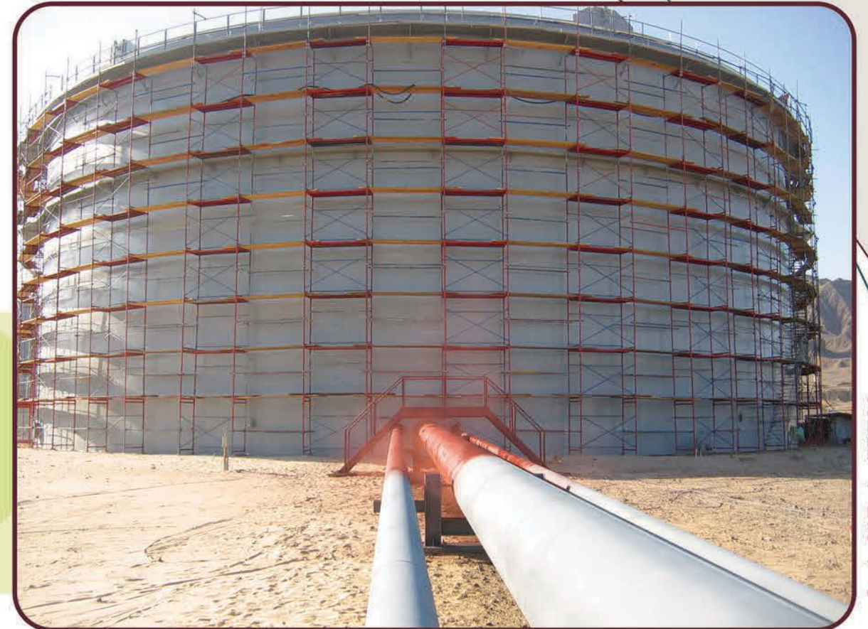
Crude Oil Tank - ZEITCO
